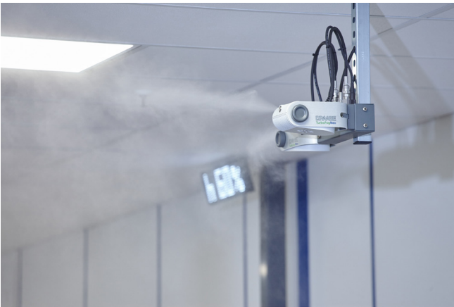
Figure 3 Example of a in-room humidifier with high-pressure nozzles. The water is atomised into a micro-fine fog at up to 70 bar and is immediately absorbed by the ambient air.
